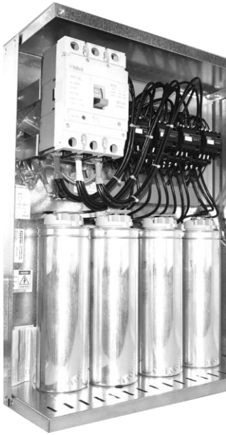
Switchable Capacitor Bank
